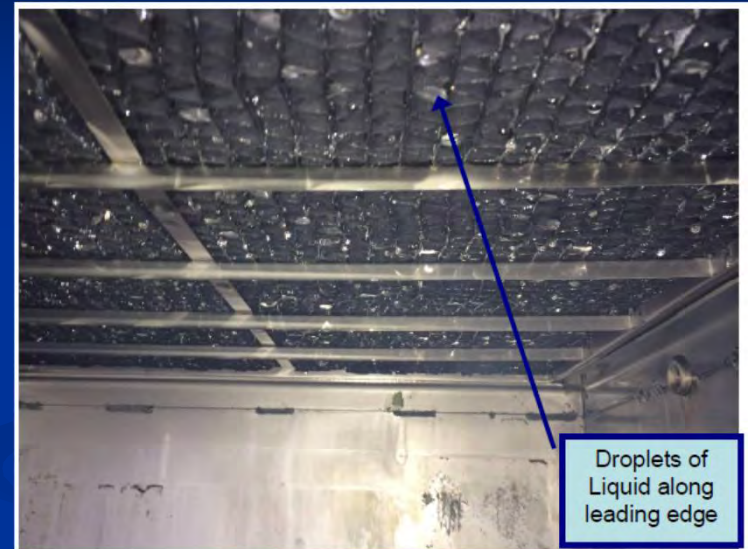
Modules in operation
